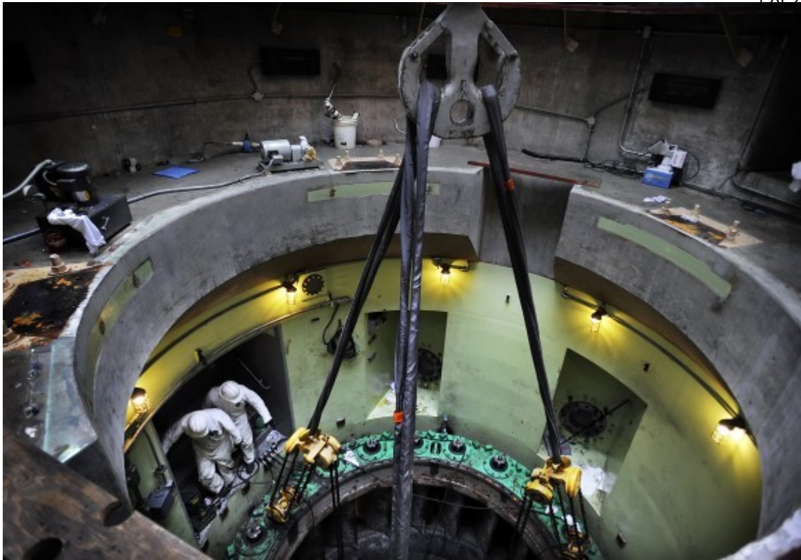
Workers at the Kingsley Dam hydro plant remove parts that will be sent out for repair Oct. 19. (JACOB HANNAH/ Lincoln Journal Star)
